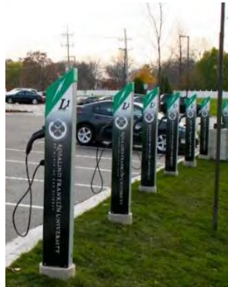
Pedestal – owner can leave personal EVSE in trunk, reduce theft
